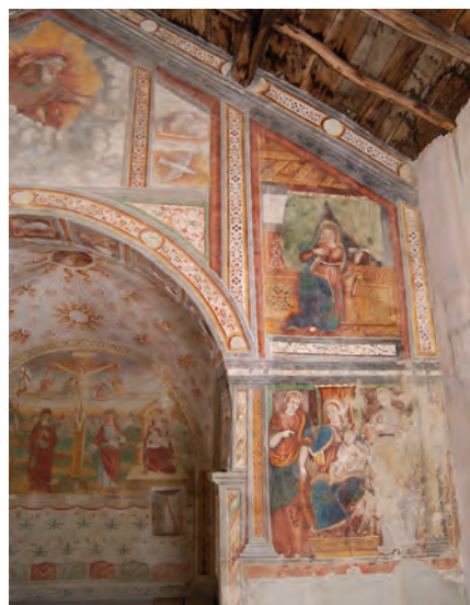
Fig. 1 - St. Alessandro church in Lasnigo (Como, north Italy), south part of the chancel arch. The blue drapes show an irregular and inhomogeneous alteration of azurite
